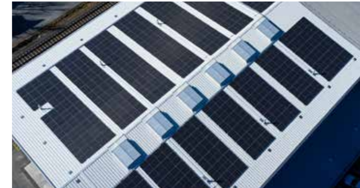
1,000 m 2 of solar panels on the production hall State-of-the-art thermal insulation glazing
